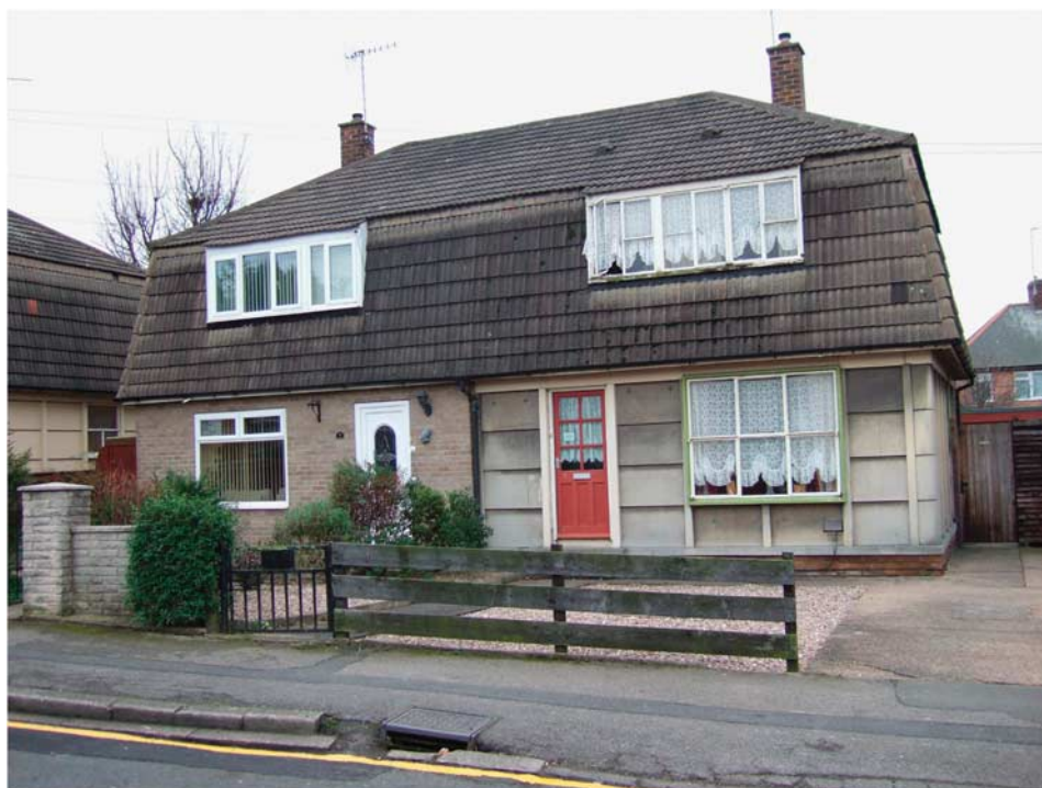
Figure 3: Different evolution of non-traditionally constructed semi-detached houses. The house still in its original form (right) requires significant refurbishment.
