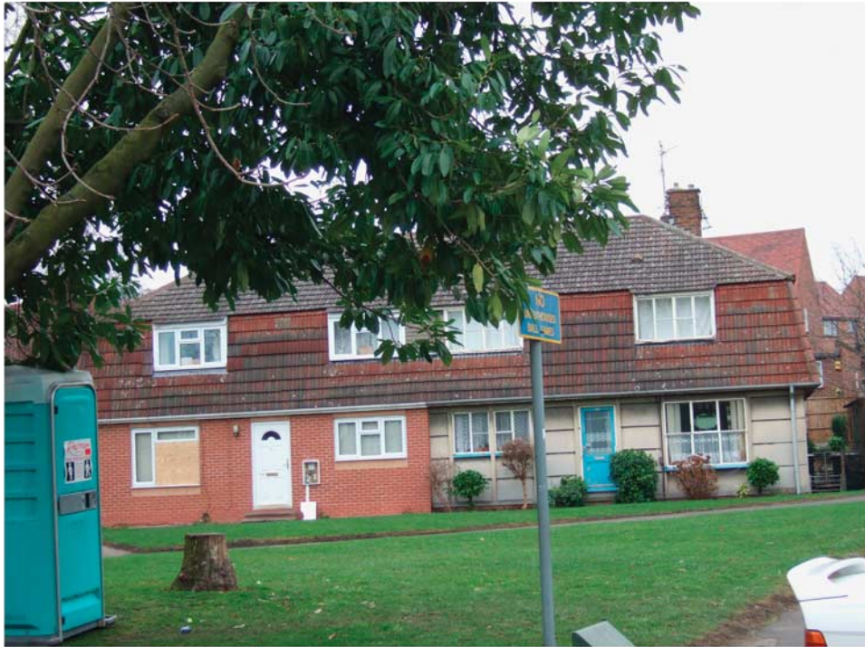
Figure 1: Original construction of small pre-cast concrete panels supported by pre-cast columns (right) and overlaid with brick (left).
